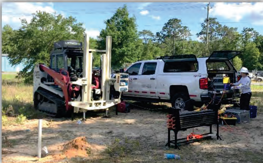
EGS Performing CPT / HPT / Conductivity Logs and Setting Cased Hole Piezometers for Infiltration Properties
