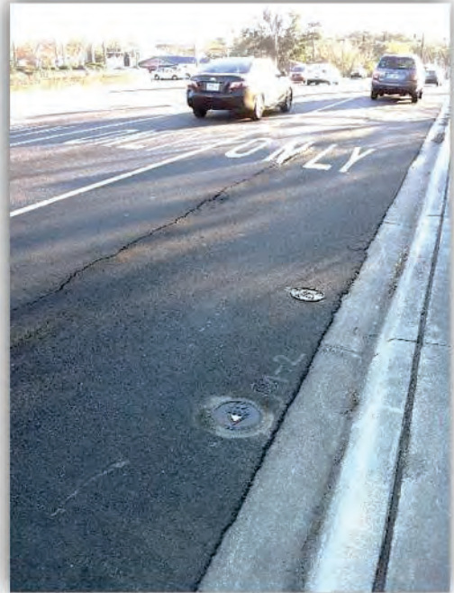
Slope Inclinometers in Roadway
